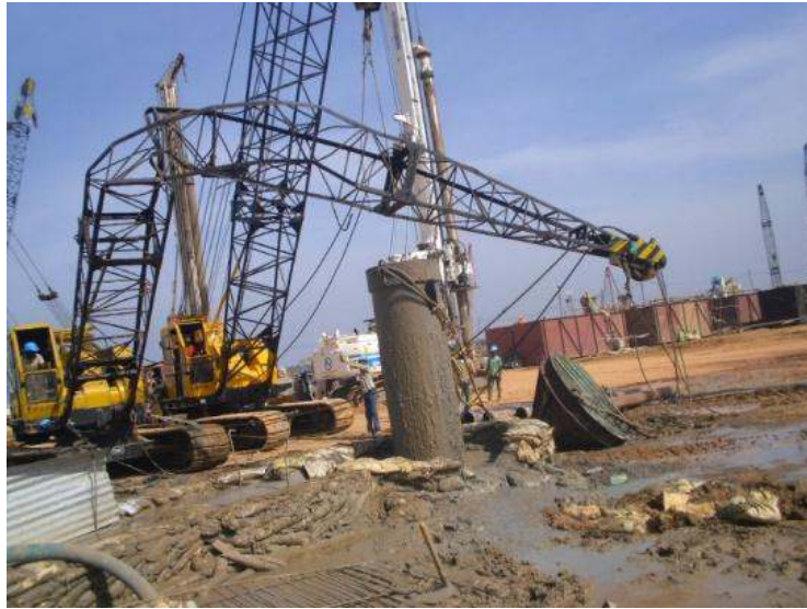
Gambar 4.78 Jib Crawler crane Patah
