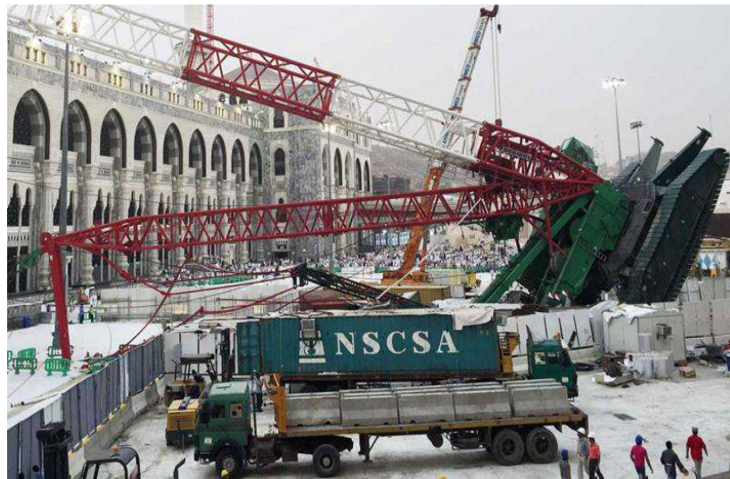
Gambar 4.80 Crawler crane Roboh
